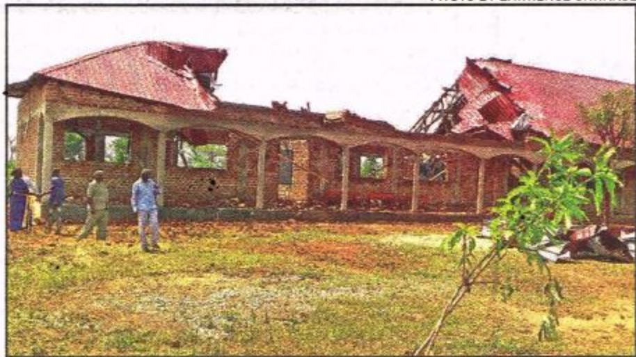
Residents and administrators inspecting a classroom block which iron sheets were ripped off by the heavy hailstorm on Saturday
