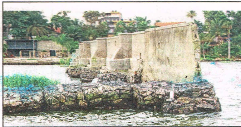
A perimeter wall of Ddungu Beach constructed in the waters of Lake Victoria at Mulungu in Munyonyo, Makindye division
