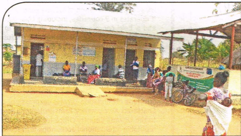
The old outpatient department block at Angagura Health Centre III in Pader district which was constructed by the Government
