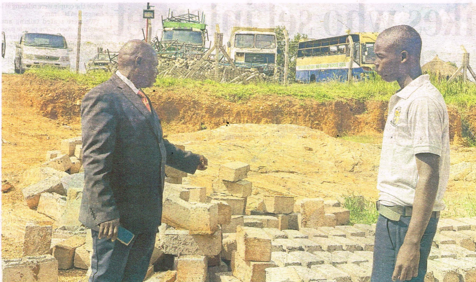
Emmanuel Arima talks to a student at the school's construction site in Arua, where classroom learning is blended with hands-on building, farming and technical training. PHOTO/PROMISE TWINAMUKYE
